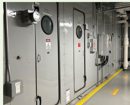
Air handling unit, Kelowna General Hospital, Canada
