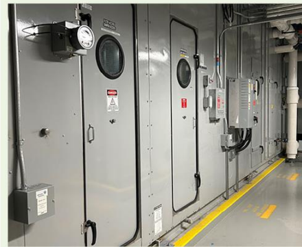
Air handling unit, Kelowna General Hospital, Canada
